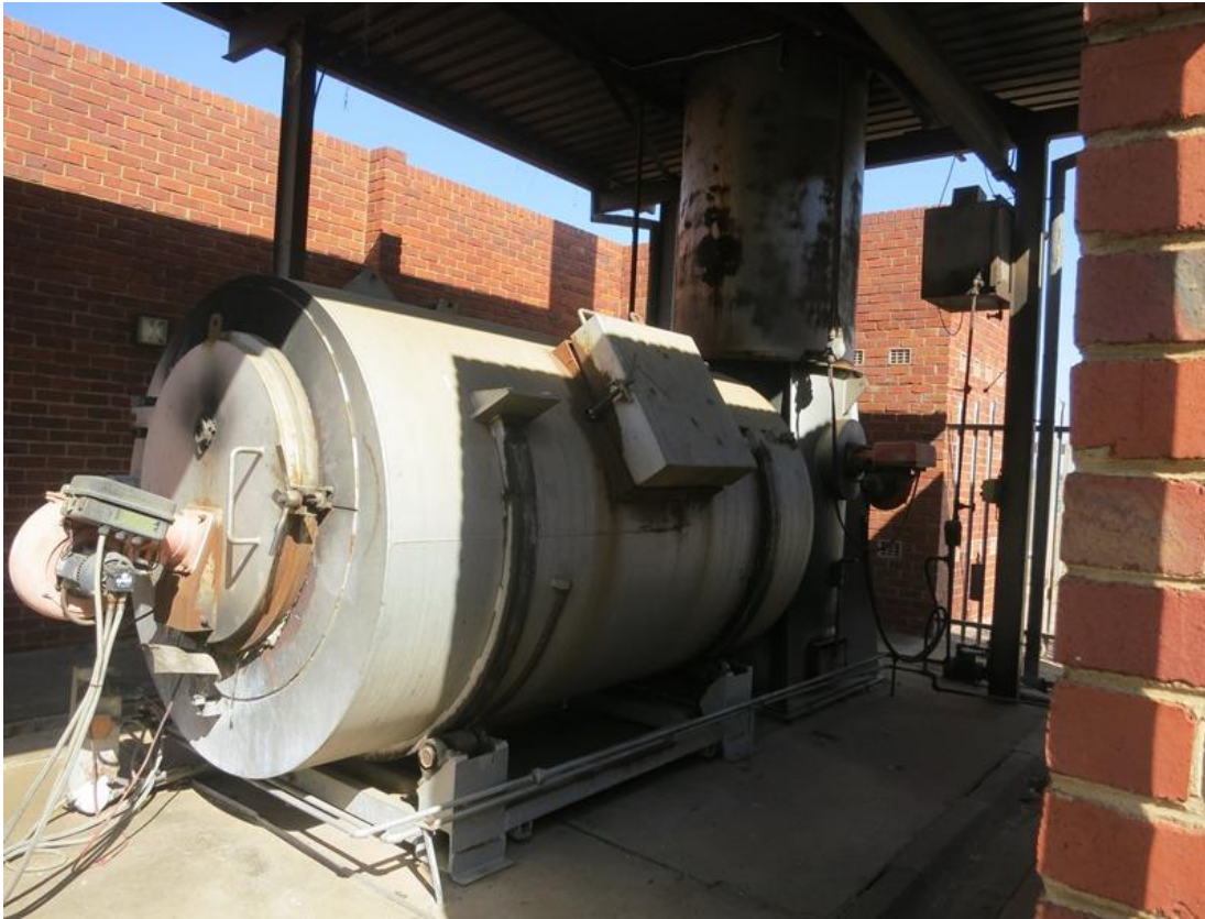
Figure 7: Another view of the incinerator.
