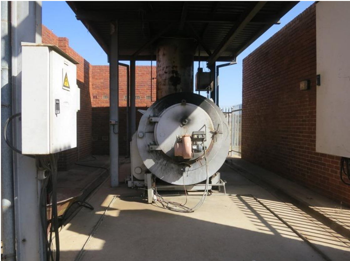
Figure 4: View of the Incinerator inside the building.
