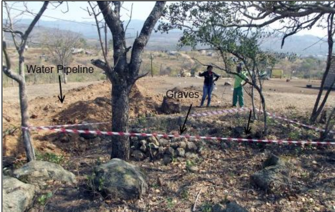
Fig. 15. Site UT 6. Two unmarked graves and the location of the water pipe. Photo taken in Western direction.
