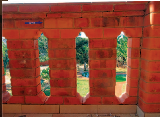
Fig. 11. The view from the upper loggia. Note the rounded bricks of the pillars.
