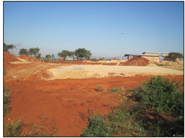
Figure 16: View of the disturbances caused by recent site preparation activities.
