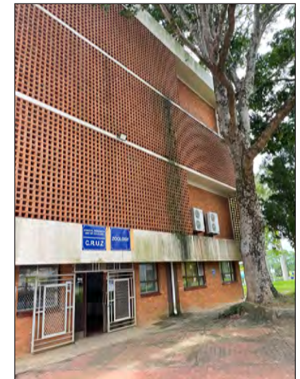
Figure 13E: Zoology building with face-brick and generic brise-soleil type of this era. (Authors own).
