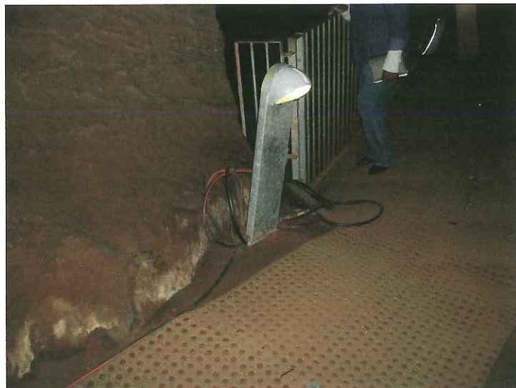
Fig 22: The inappropriate lighting (and rubber matting) on the tourist route through the Sterkfontein caves. Electrical cables and transformer boxes need to be concealed or disguised. The excess cabling is unsightly besides being a safety hazard at foot level
