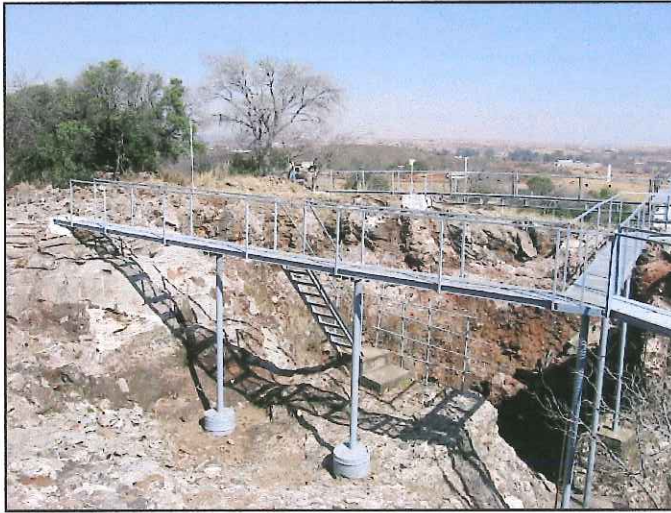
Fig 7: The current excavation area, occupying much of what was once known as the 'Extension Site', now excavated to a depth of some 9-10 metres at its deepest points. The metal walkway provides easy access to different sectors of the ongoing excavation.
