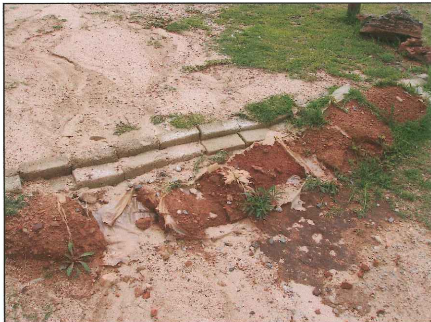
Fig. 5: Ruptured sandbagging on entrance pathway, Wonder Cave
