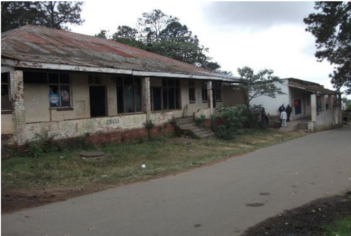
Figure 6: Unused and dilapidated building with post office in background
