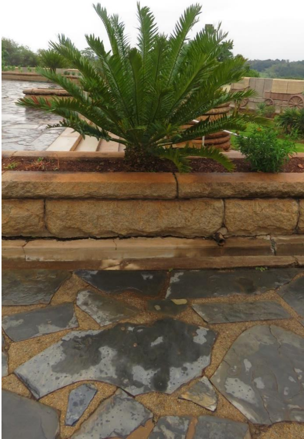
Figure 40: Note cracks in flower pots.
