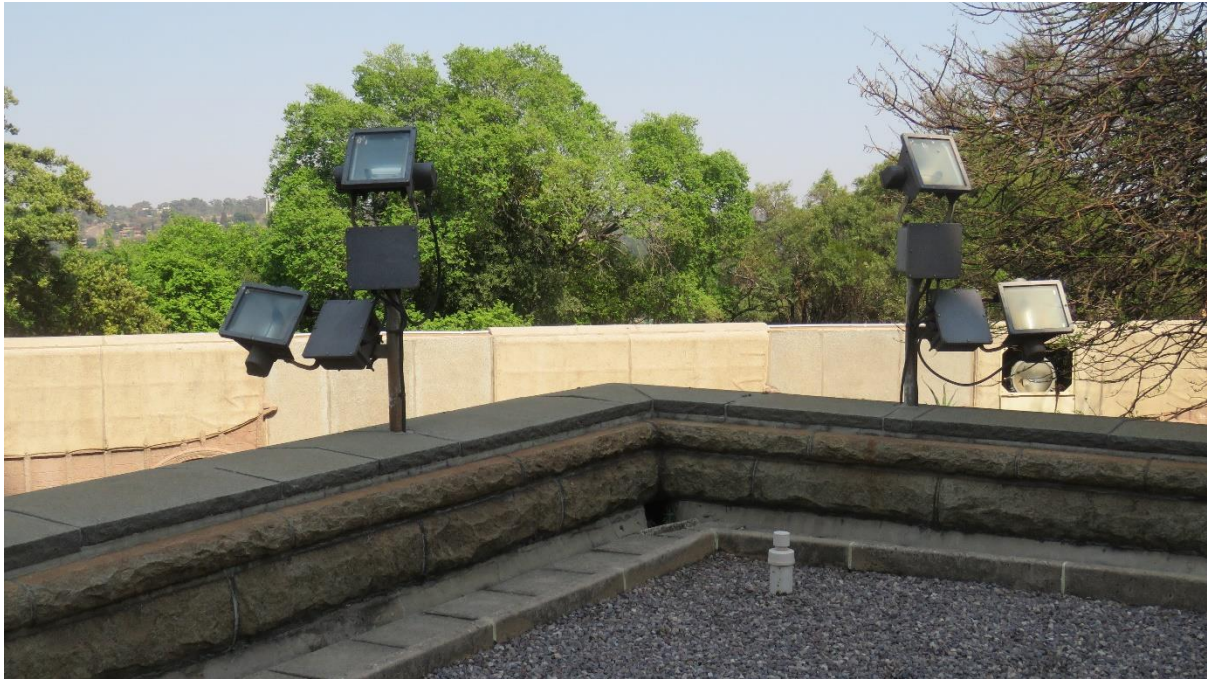
Figure 42: Example of spotlights to be replaced.
