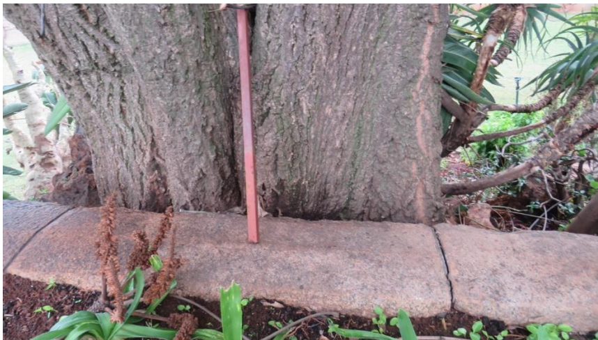
Figure 41: Tree next to flower pots that will eventually crack the pots. It needs to be removed.
