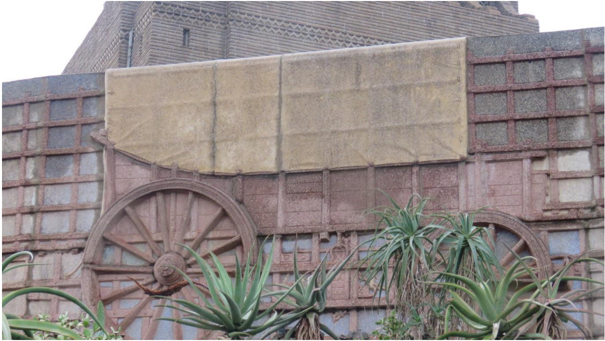
Figure 45: Section of the wagon laager showing cracking.
