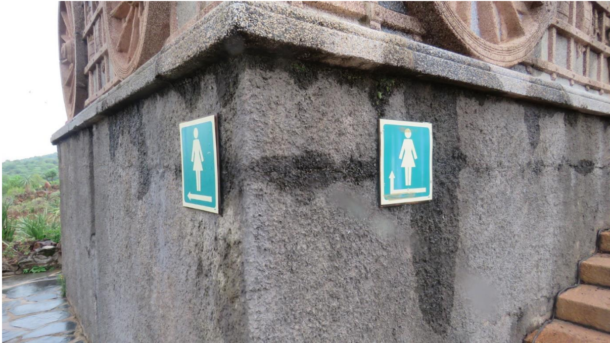
Figure 49: Wall of toilet facilities to be repainted. Also note signage that will be placed more appropriately.
