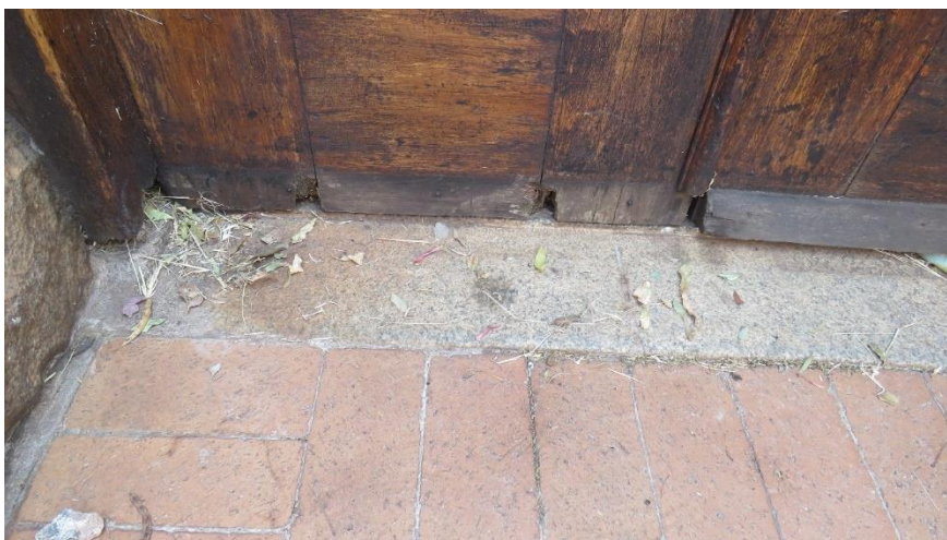
Figure 30: Note damage to the door caused by naturel weathering.
