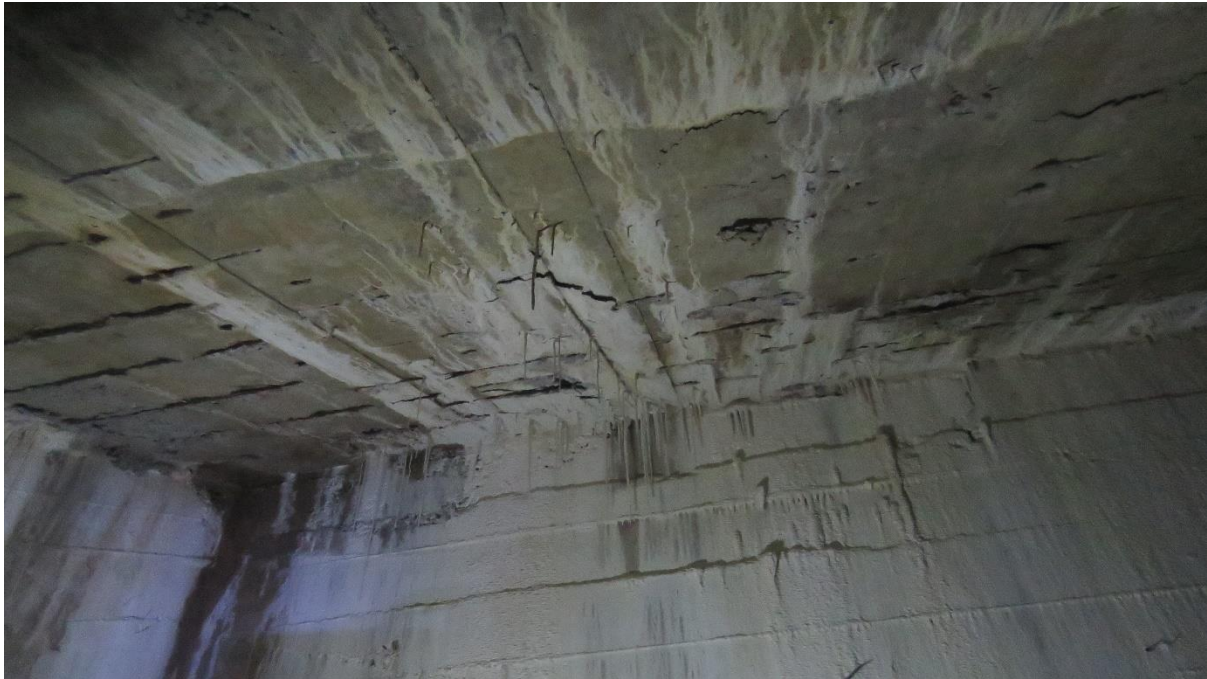
Figure 38: Note cracks and the forming of stalactites due to waterproofing issues.
