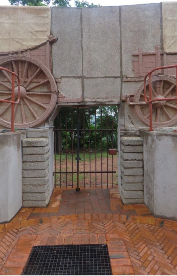
Figure 47: Sagging section of the wagon laager above the disabled entrance.
