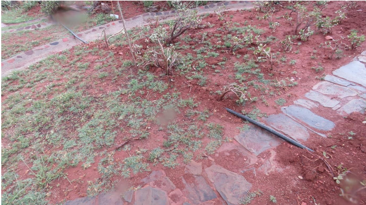
Figure 61: Example of water pipes that should be re-laid to run underneath the historical features.
