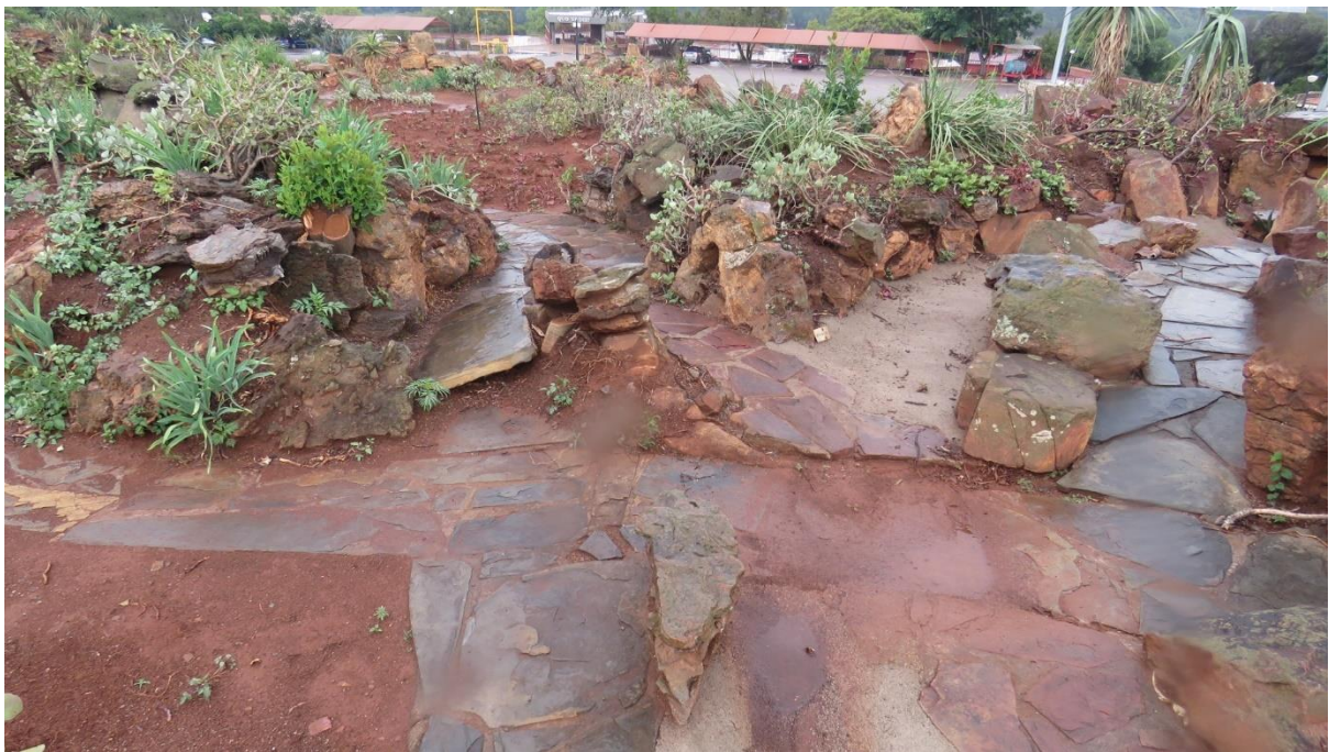
Figure 58: Example of tree stump causing damage to slate route.
