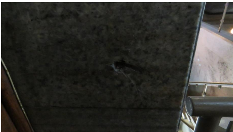
Figure 28: Granite doorframe, indicating that there once was a security door installed. This will be replaced.
