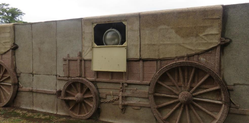
Figure 48: Example of spotlight at wagon laager to be replaced by energy efficient lights.
