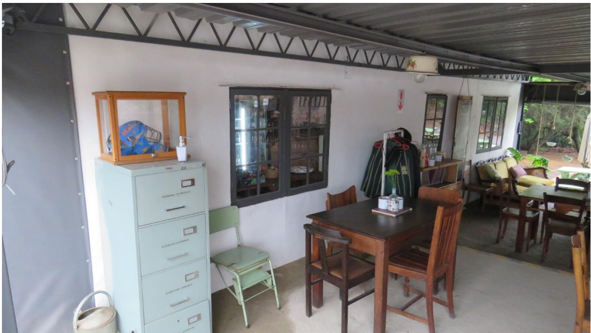
Figure 91: Front of school with loose roof and floor for customers.
