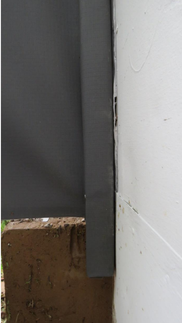
Figure 93: Loose panel with canvass next to the school.
