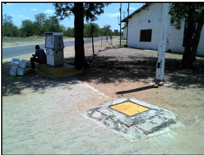
Figure 9. Current pump and underground tank.
