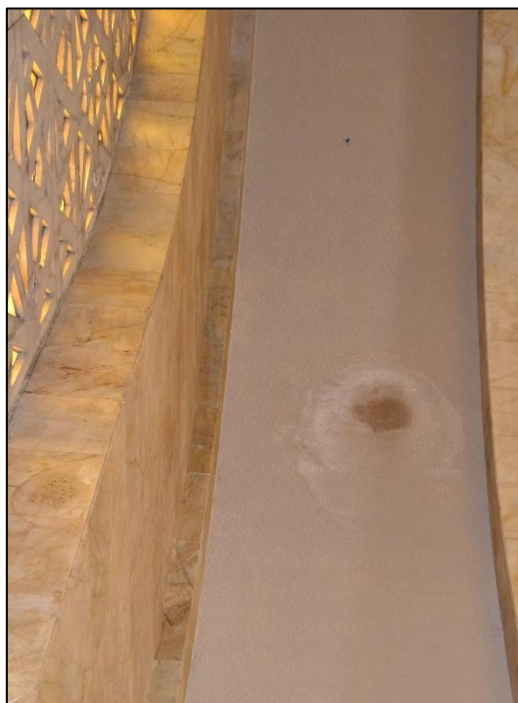
Figure 10. Close-up of the patch on the curved ceiling in the south western corner (Photograph: M. Naudé 2020)
