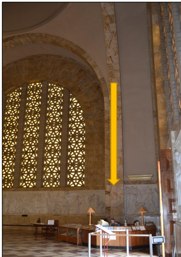
Figure 1. Location of work station of staff member in relation to arch clad with marble panels (Photograph: M. Naudé 2020)
