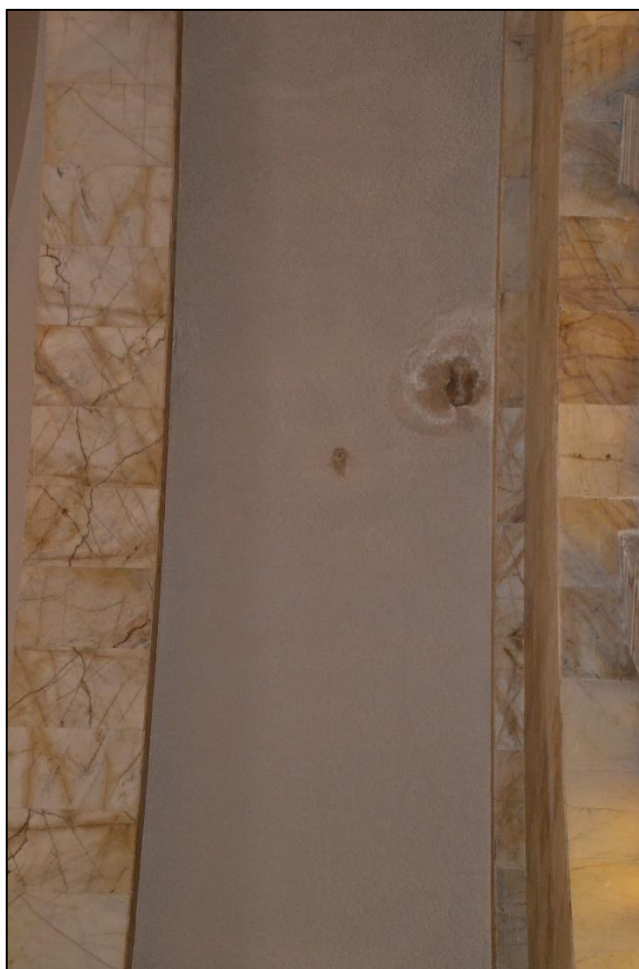
Figure 6. Second set of dark patches where moist degraded the plaster along the arched ceiling of the southern elevation (Photograph: M. Naudé 2020)
