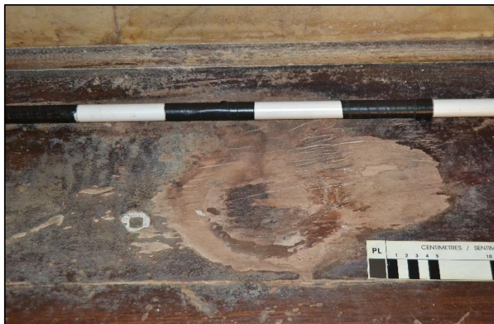
Figure 5. Dripping water has damaged the wooden seat surface (scale bar sections – 10cm long) (Photograph: M. Naudé 2020)
