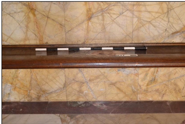
Figure 4. Moist has been dripping on the wooden seats along the wall of the southern side of the interior (scale bar 1 m long) (Photograph: M. Naudé 2020)
