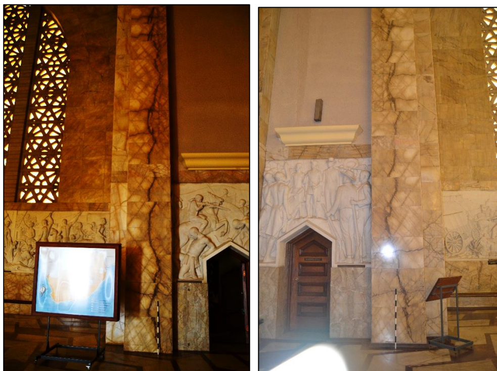
Figure 12. Vertical cracked marble panels along the intrados of two corner arches (Photograph: M. Naudé 2020)
