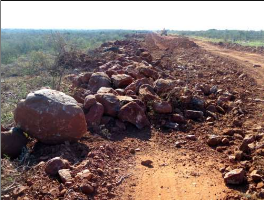
Figure 9: Displaced andesitic boulders along the W-E sector of the main access road (Loc. 330). The bedrocks here are igneous and therefore not fossiliferous.
