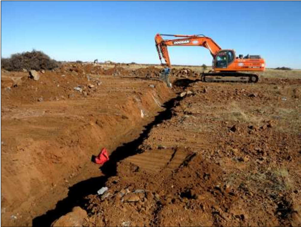
Figure 11: In some areas shallow trenches for underground cables in the PV panel array areas mainly intersect gravelly soils (Loc. 029).
