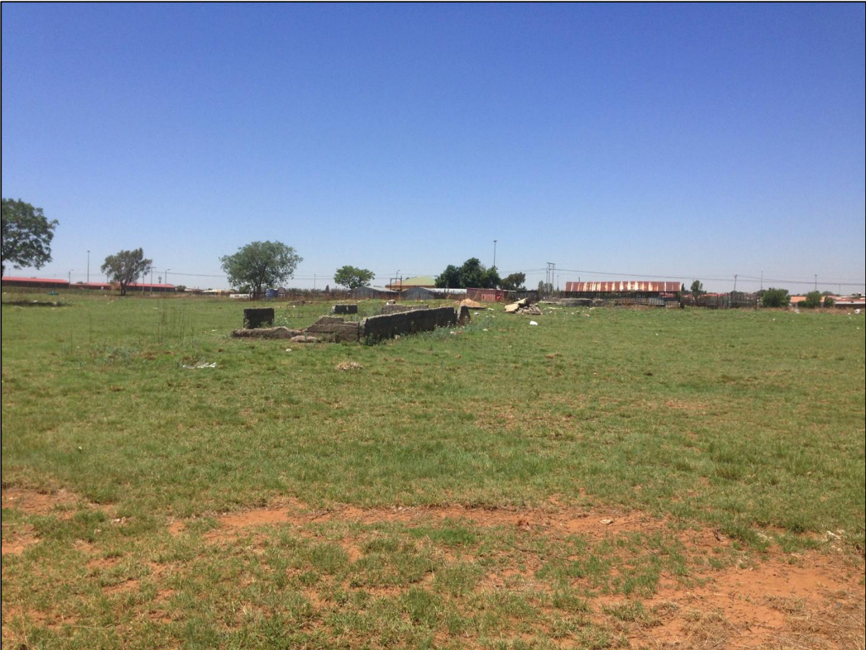
Figure 4. Foundation remains and dilapidated structures on site
