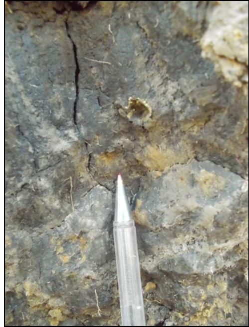
Note: Desiccation cracks in profile.
