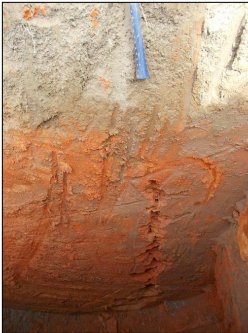
Note: Hole stopped TLB soft excavation.
