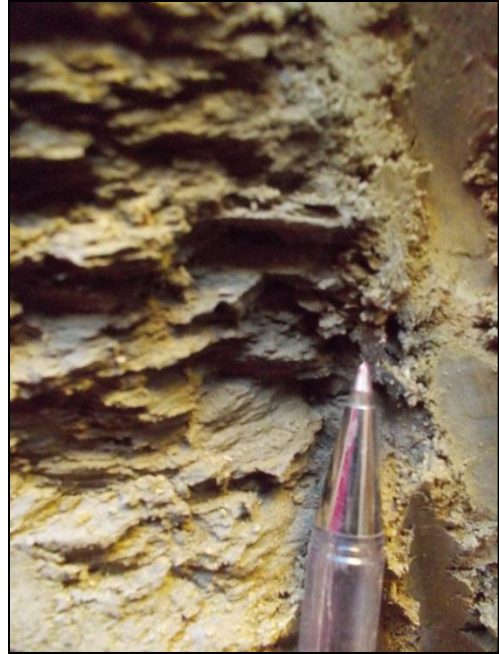
Note: Layered structure in highly weathered shale.
