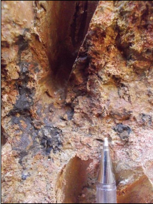
Note: Iron and manganese staining.
