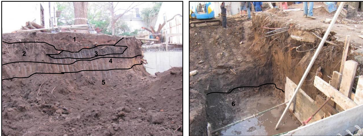
Plate 11: View of the east wall of the excavations for the parking garage; Plate 12: View of the excavation some 3m from the surface, showing the river cobbles and water table.
