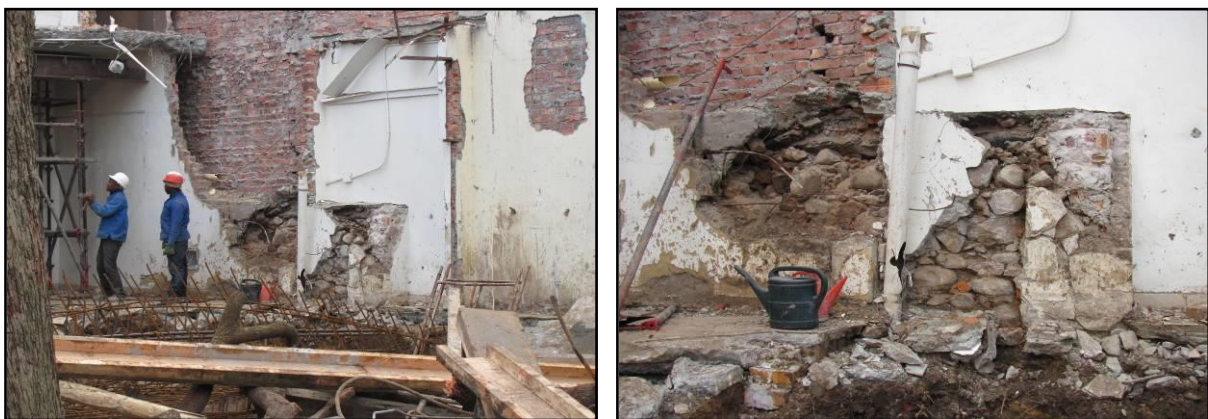
Plate 13: View of the north boundary of Erf 1261 and the southern boundary of Erf 1258. Note the section of stone walling abutting the red brick wall. Plate 14: Close up of the stone walling.
