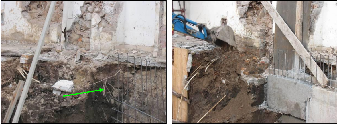
Plate 15: Note the stone walling continues below ground level for a further 1.5m. Plate 16: After the wall started to collapse, a portion of concrete had to be cast to retain the lower section.
