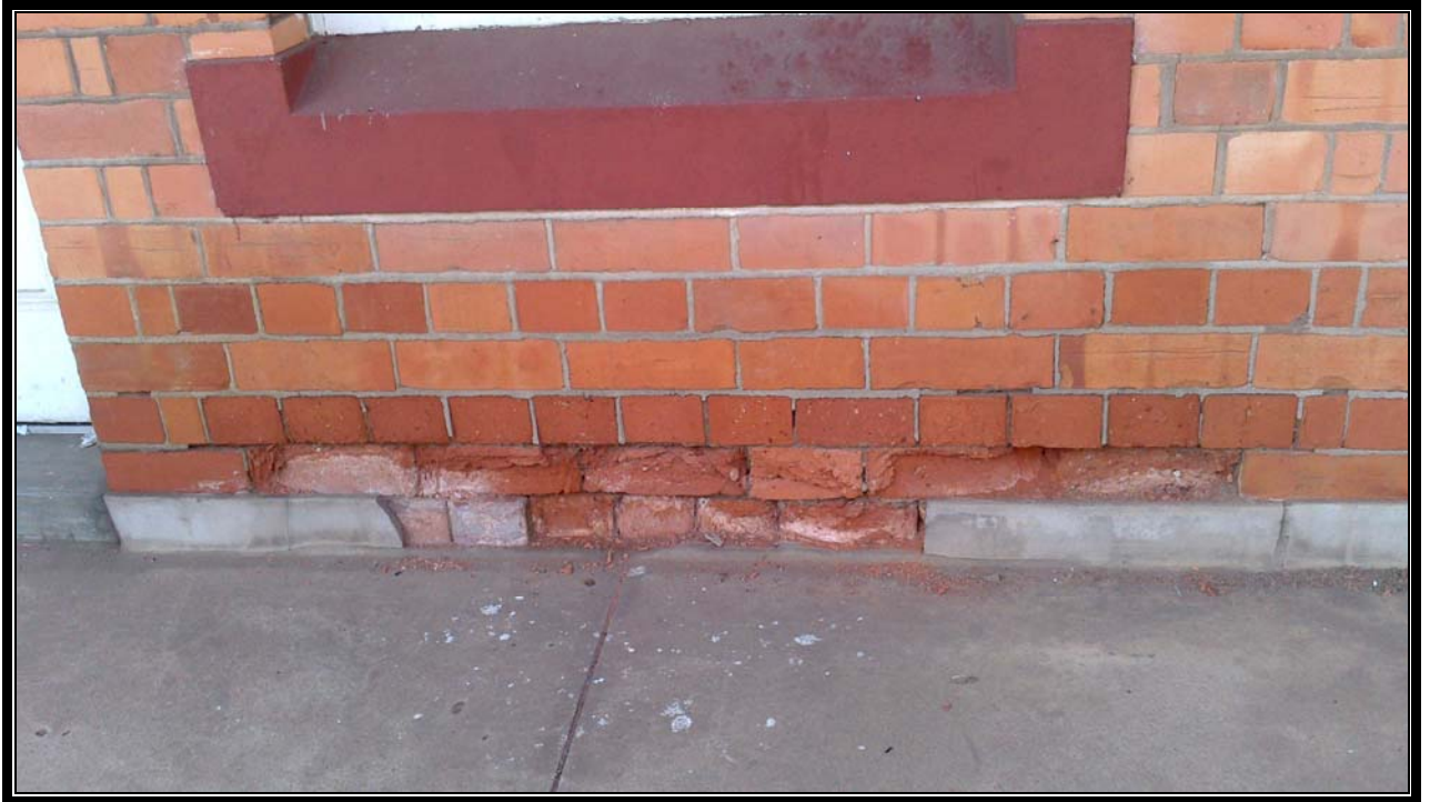
Photograph 5: View of damaged brickwork along entrance wall of Larger building.
