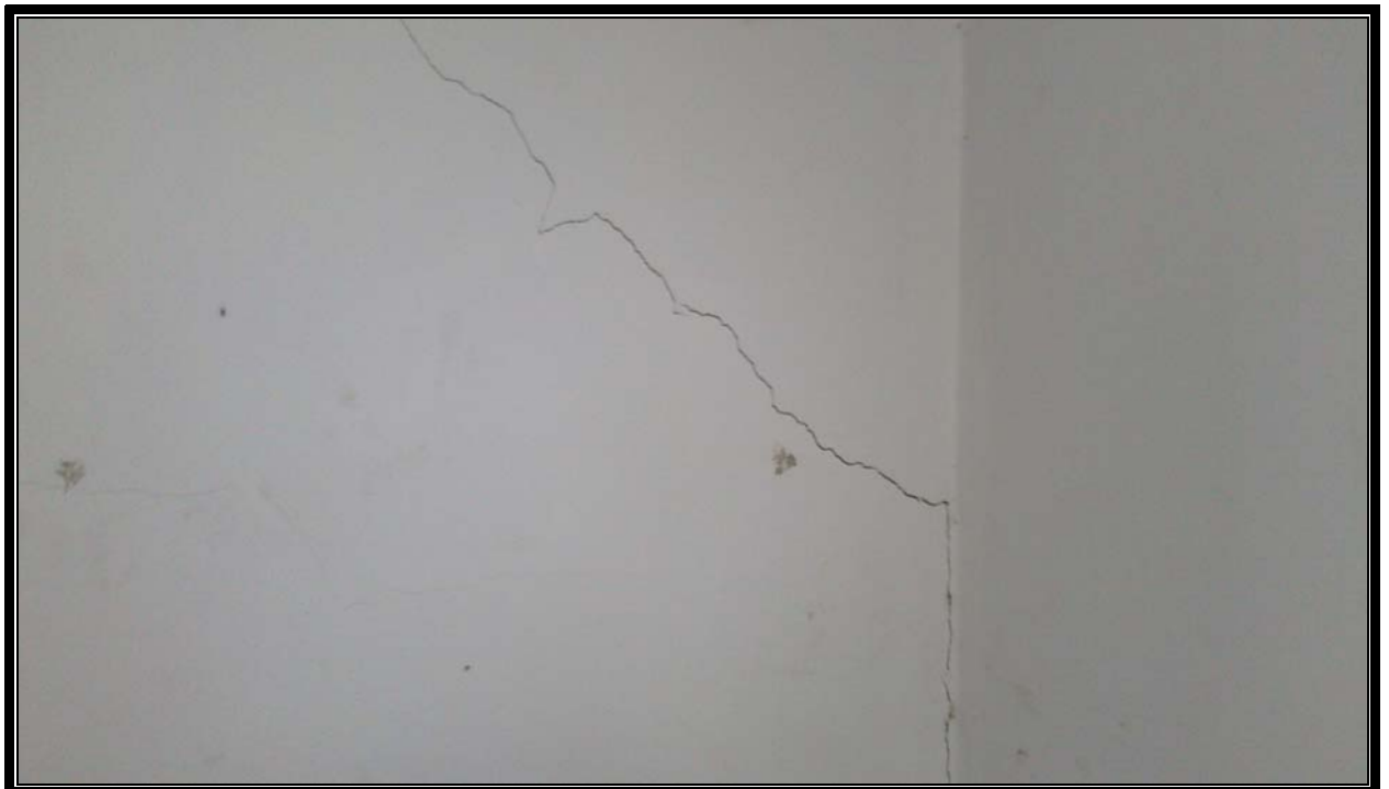
Photograph 4: View of Crack along rear Wall of Larger building
