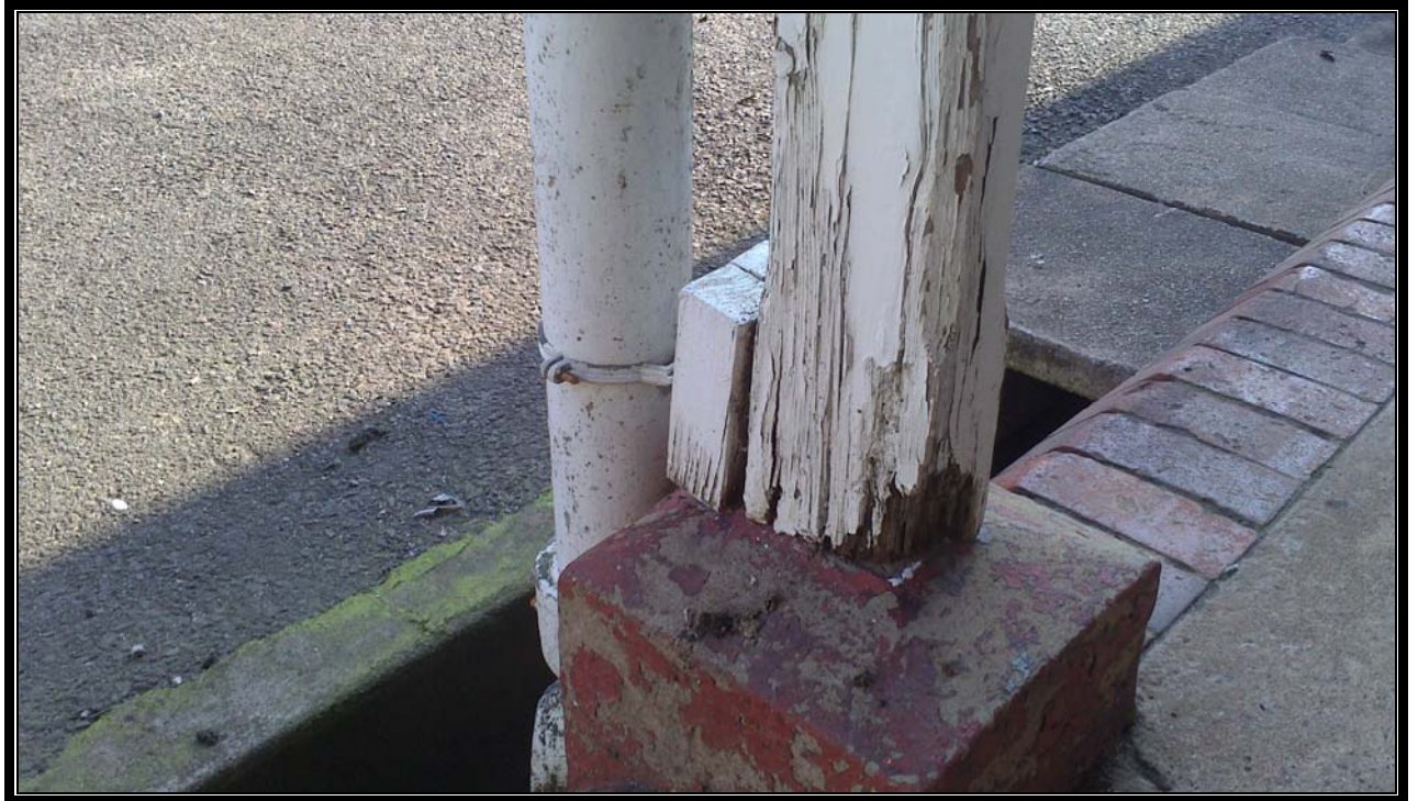
Photograph 7: View of damaged and deteriorated verandah post
