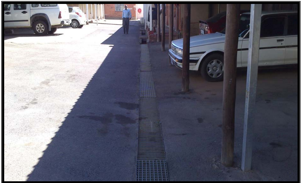
Photograph 12: View of channel (grating over) used to convey Stormwater away from Buildings. Channel observed to be blocked and requires cleaning.
