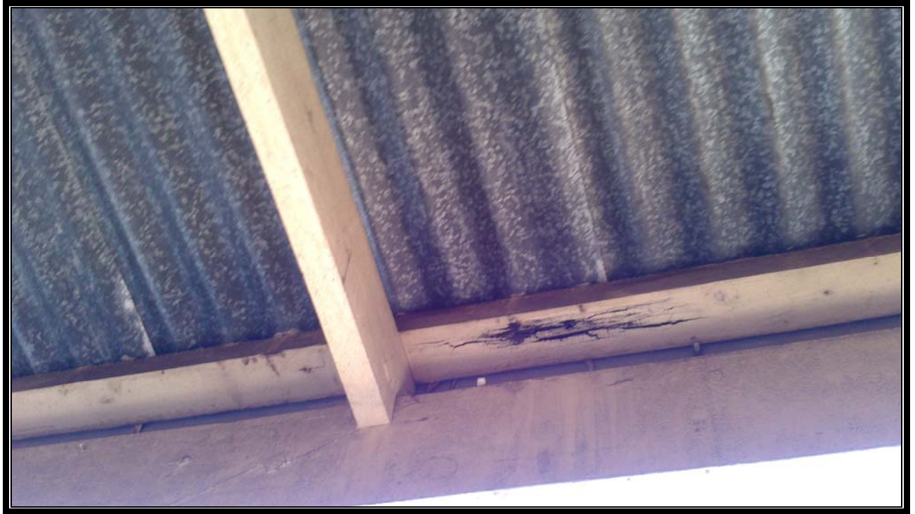
Photograph 9: View of deteriorated verandah purlin.
