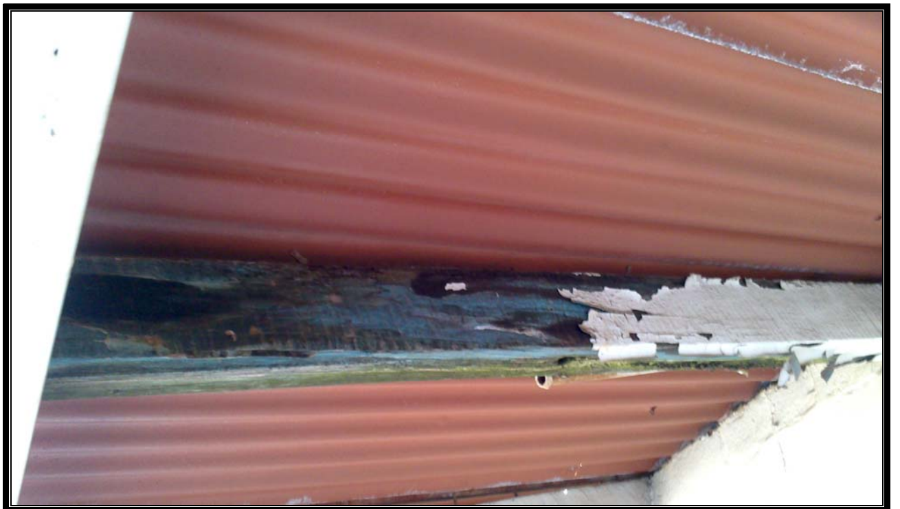
Photograph 10: View of deteriorated verandah rafter
