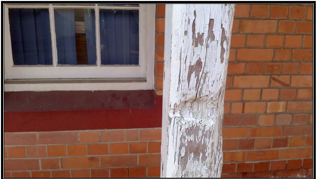
Photograph 6: View of damaged verandah post
