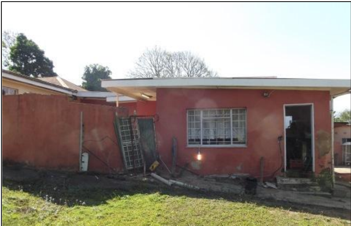
Fig. 2. Site WAH 1. Photo of the attached house on the Southern side of the original.
