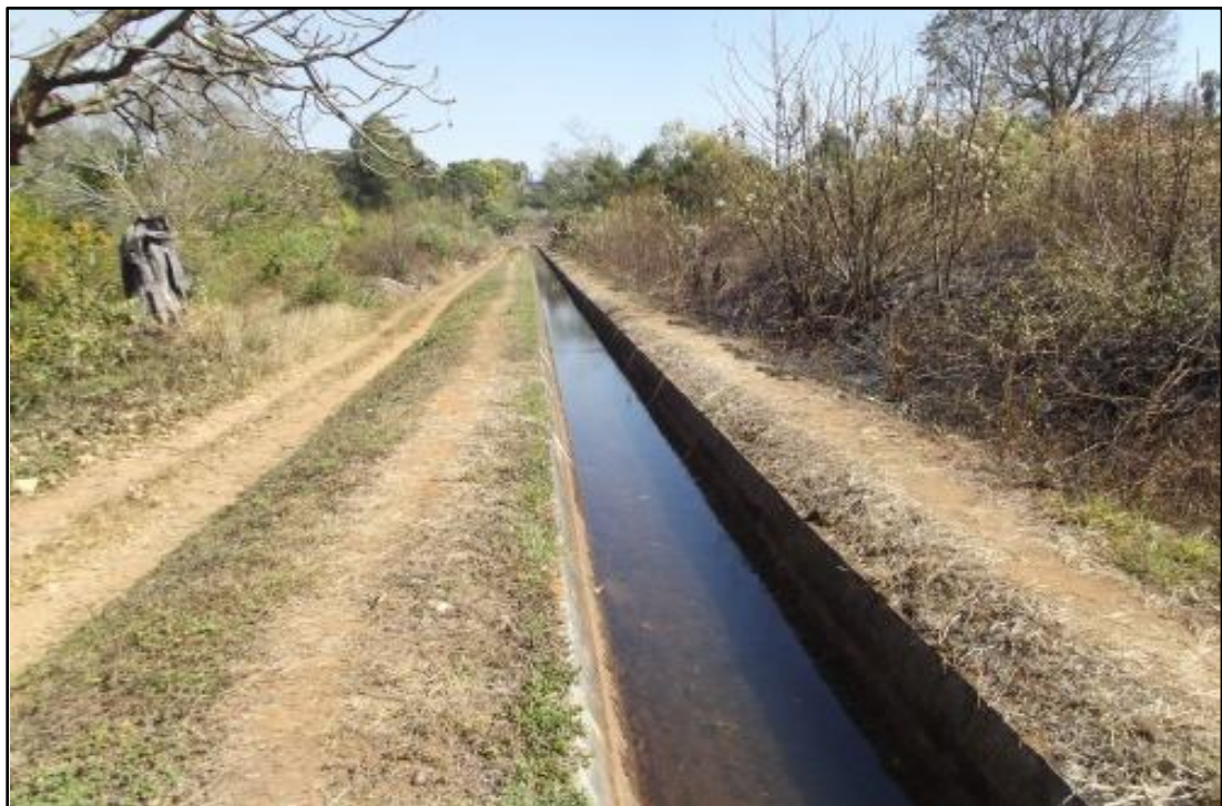
Fig. 8. WAH 4. A section of the historic water canal. Photo taken in Western direction.
