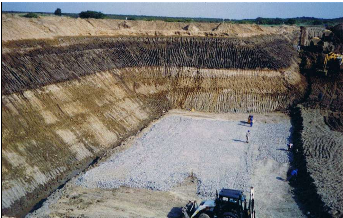
Figure 3. Excavations at Berth 306, Richards Bay Harbour. Exposure of Cretaceous horizons at 14m below m.s.l.
