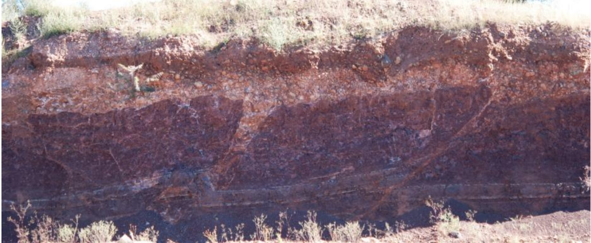
Figure 12: Borrow pit 1: Burgersdorp Formation mudstones showing 3 metre deep faults filled with geologically recent calcretised pebbly deposit.
