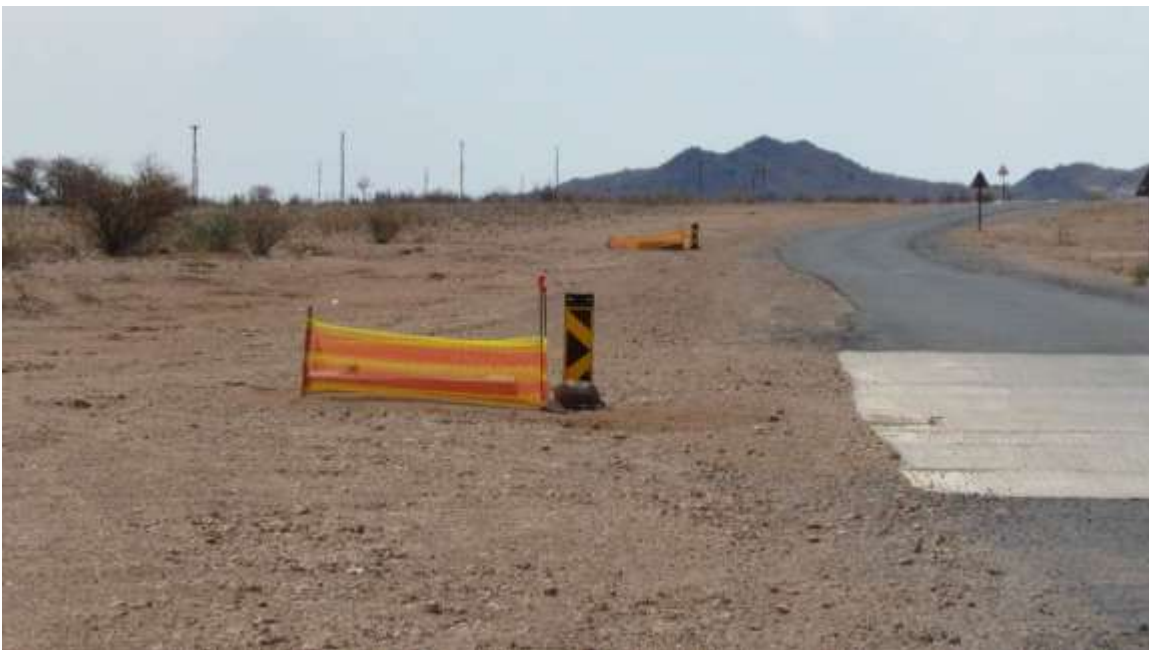
Pipeline route within the road servitude, subject to prior disturbance in road construction.
