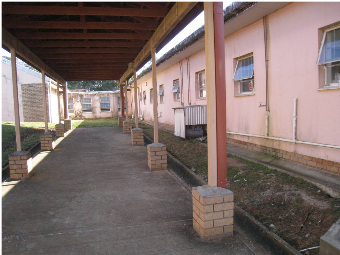
Fig 32: Rear of the junction of the Outpatients Block (right) and junction with the Physiotherapy Block (centre)
