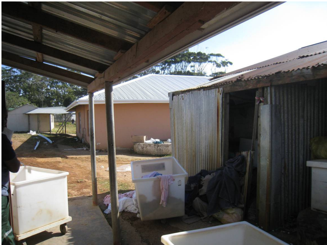
Fig 28: The Laundry Block veranda looking towards the rear extension of the Administration Block with the Old Stores to the right
