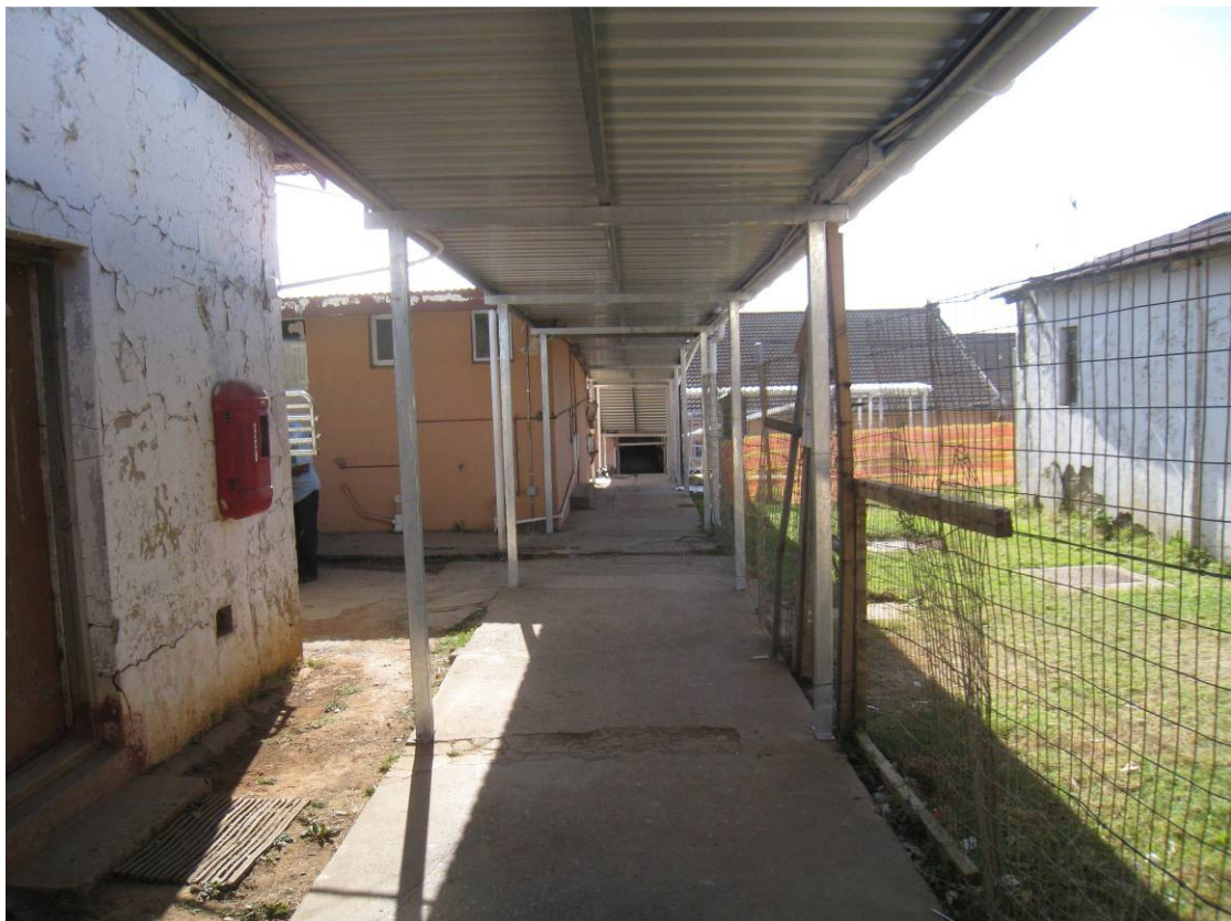
Fig 12: View down hill from Laundry and kitchen – store to the left, Administration Block jutting into the view, the Physiotherapy Block in the distance and the old Matron’s Accommodation to the right
