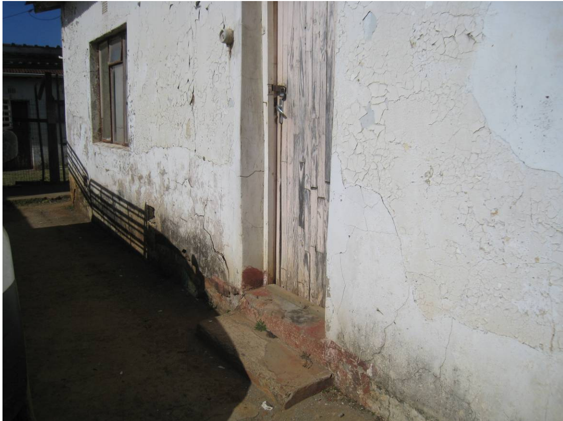
Fig 26: The Old Stores building showing the condition at ground level as well as the general wall condition
