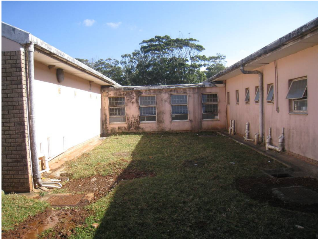
Fig 42: View of connecting passage between Outpatients Department on the right and the Physiotherapy Block on the left. Note damp issues on all three structures.
