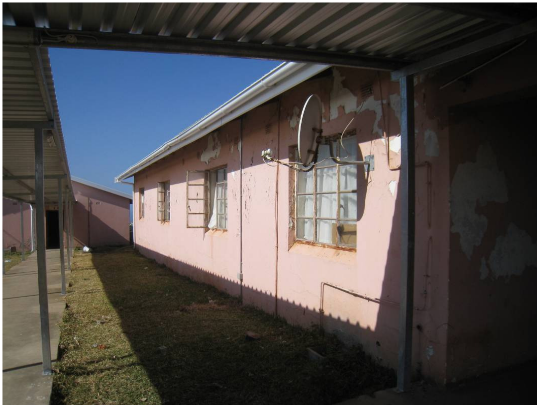
Fig 38: Staff accommodation showing condition of building as a result of lack of maintenance and damp.
