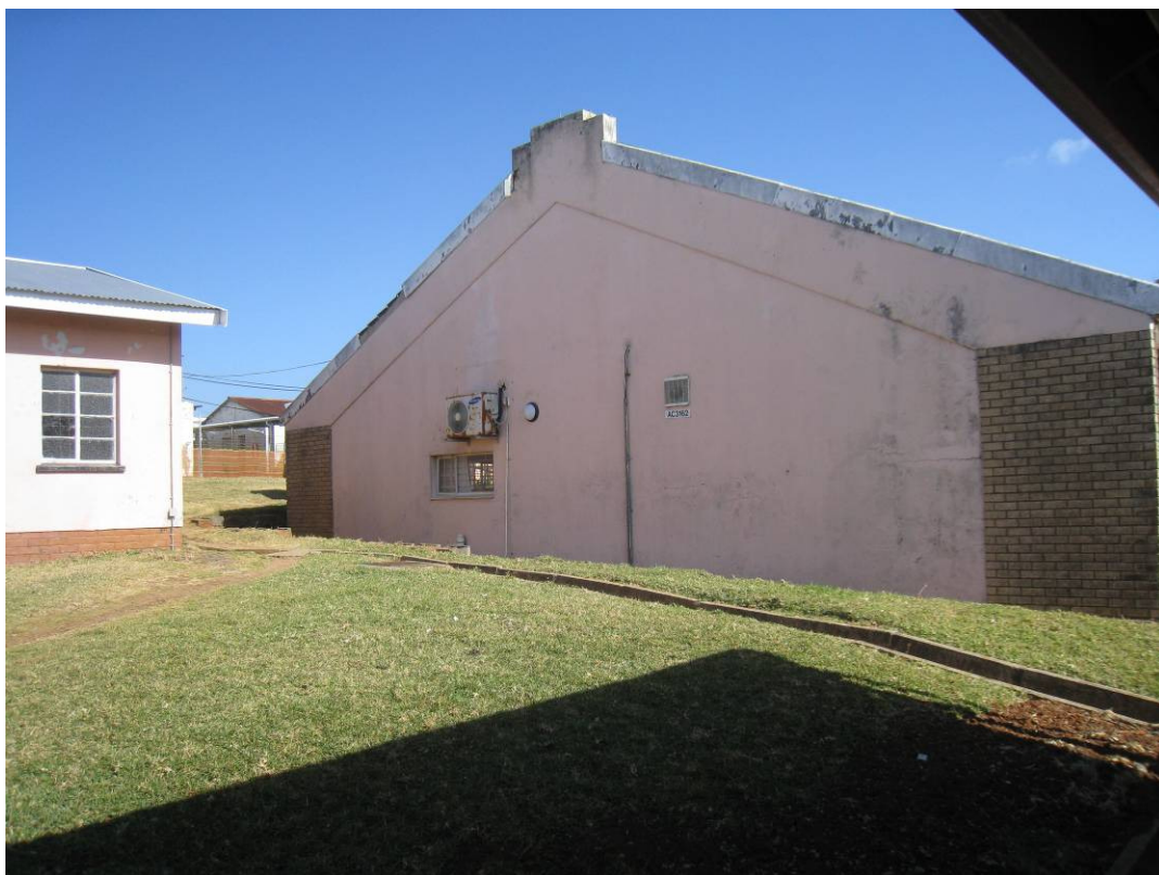
Fig 43: View of Physiotherapy Block from the north east with the end of one of the Nurses Accommodation buildings to the left. Note water incursion both from above and below.
