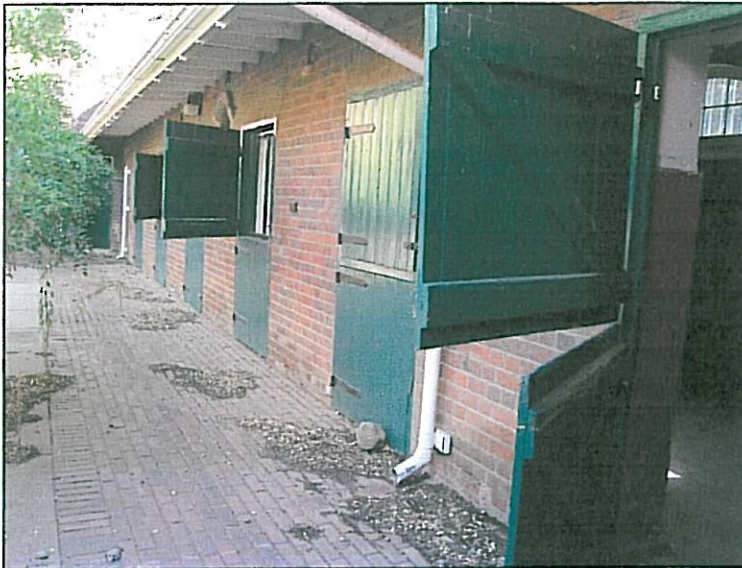
Fig.6 The building and stable doors are still in good order.
