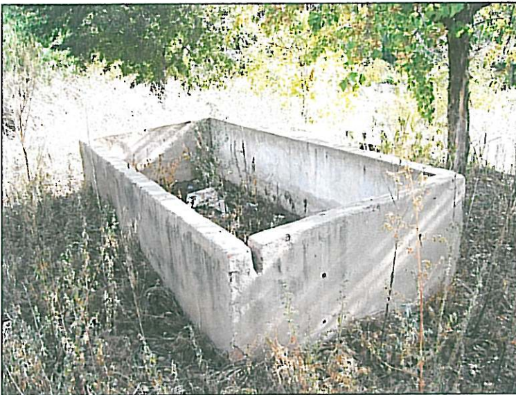
Fig.53 This concrete feature known as a "mist-propagation bed", part of the PWD nursery.
