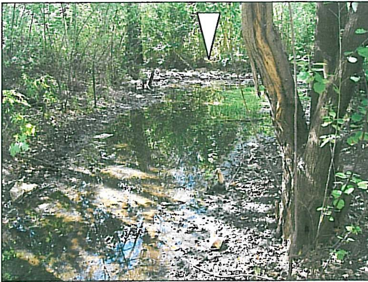
Fig.52 Rainwater forms a permanent pool against the old dam wall.
