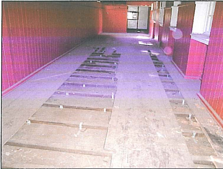
Fig.8 The extent of the vandalism is becoming serious.
