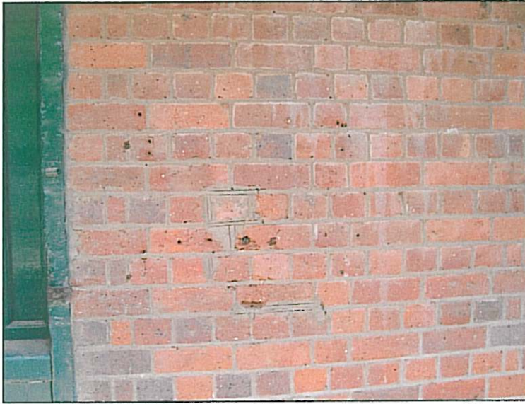
Fig.12 Position of the National Monuments plaque possibly removed by vandals.
