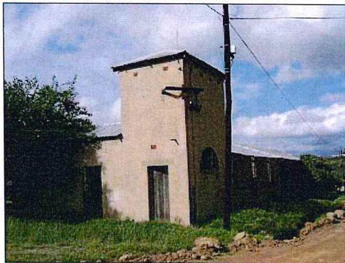
No 1d: Pumphouse and reservoir (to be preserved), with No 3c (left): Face brick store
