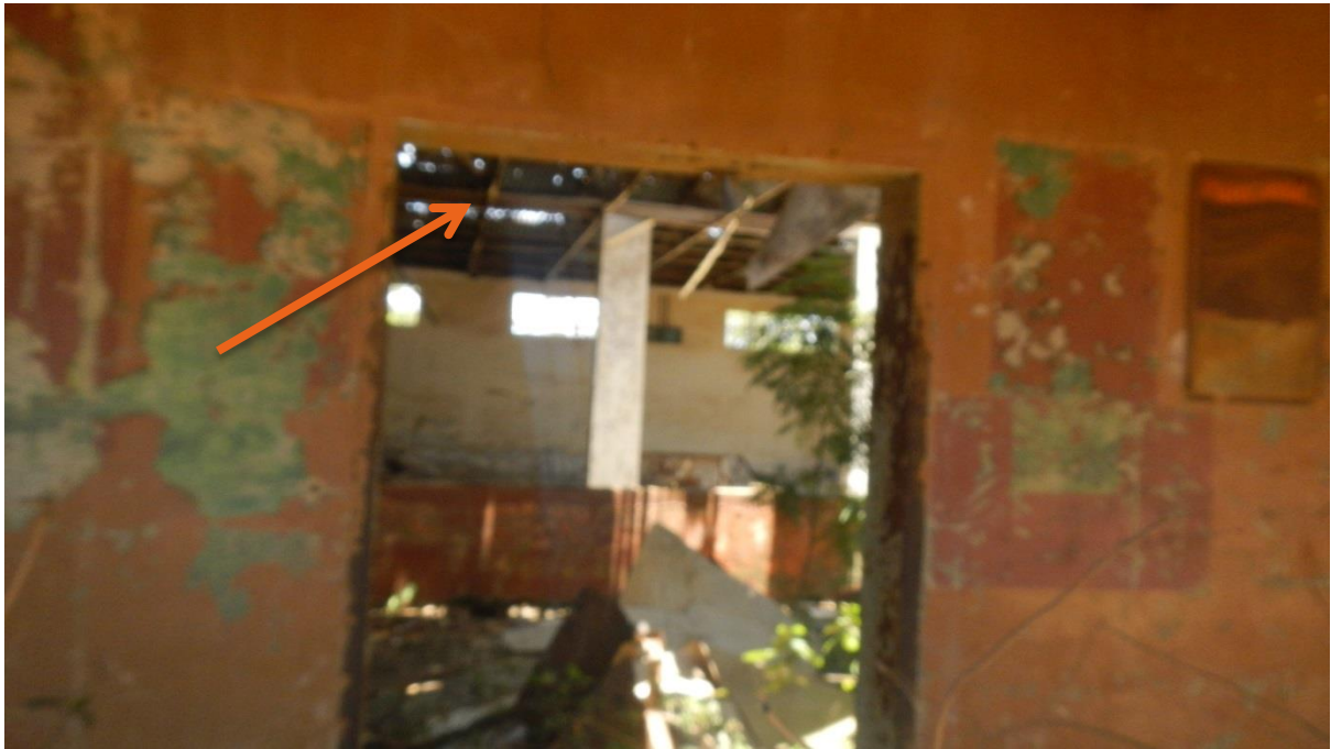
Figure 10: View of the fallen ceiling from the outside
