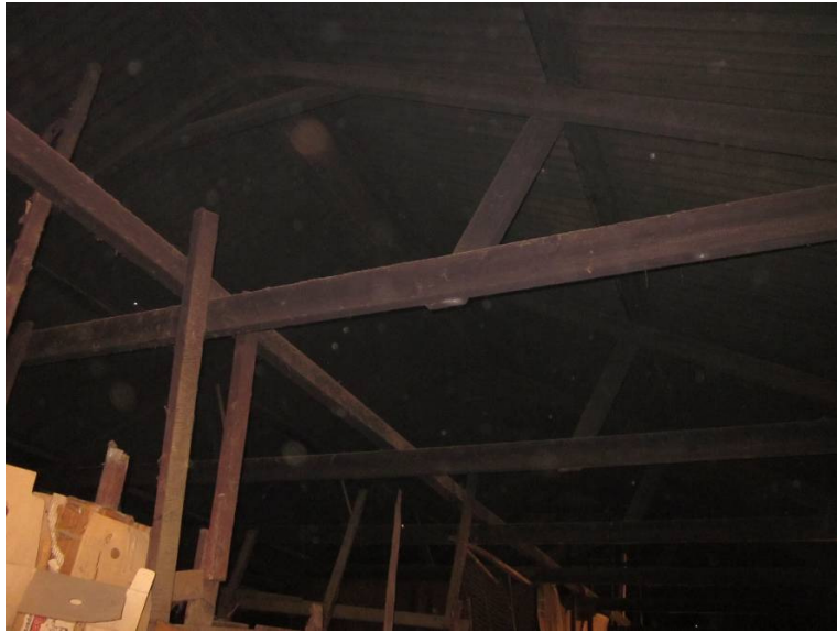
Fig 14: Trusses in roof space – note ad hoc additions in terms of space dividers
