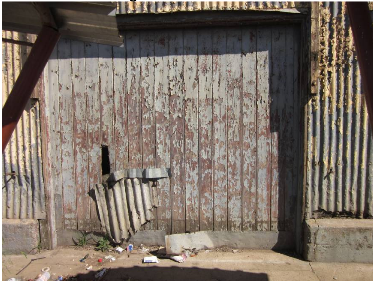
Fig 10: Showing sliding timber door, patched
