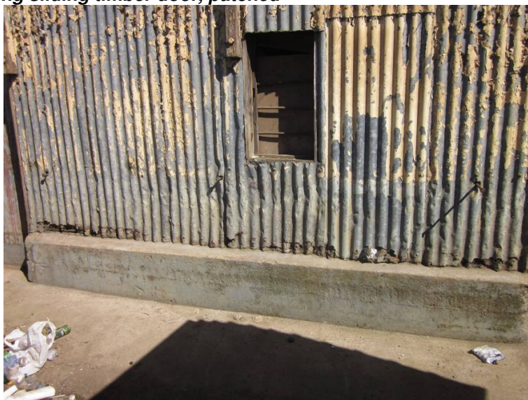
Fig 11: Base of wall adjacent to door (above) with concrete plinth
