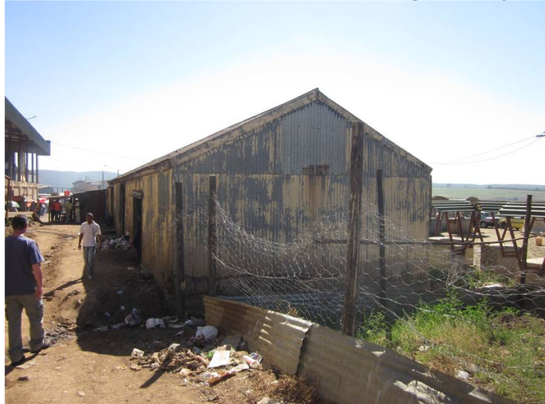
Fig 13: View of south elevation looking down the space between the large building to the west and the western elevation
