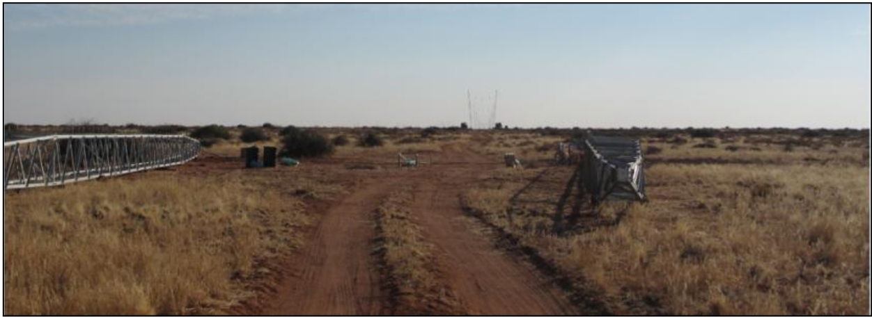
Figure 7: View northwards along the north-western margin of the study area showing a new power line currently under construction (during July 2017) parallel to part of Alternative 1.
