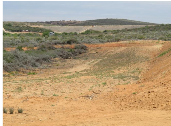
Figure 15: Smaller Scheepersvlakte Dam under construction immediately south of the proposed dam site
