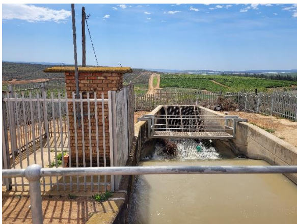
Figure 14: Existing siphon off-taking from Kirkwood Primary Canal similar to the proposed siphon infrastructure
