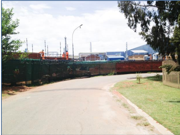
Photograph E-1: Brick wall under construction around the PMR boundary adjacent to Mey Street
