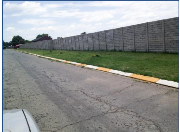
Photograph E-2: The concrete fence erected along Stobart Street around the East Geduld Club
