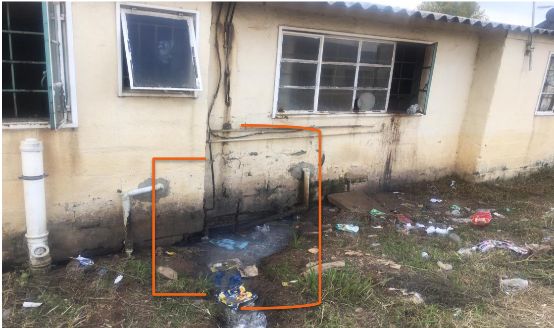
Figure 4 : Broken sewerage pipes lying in the midst of the hostels
