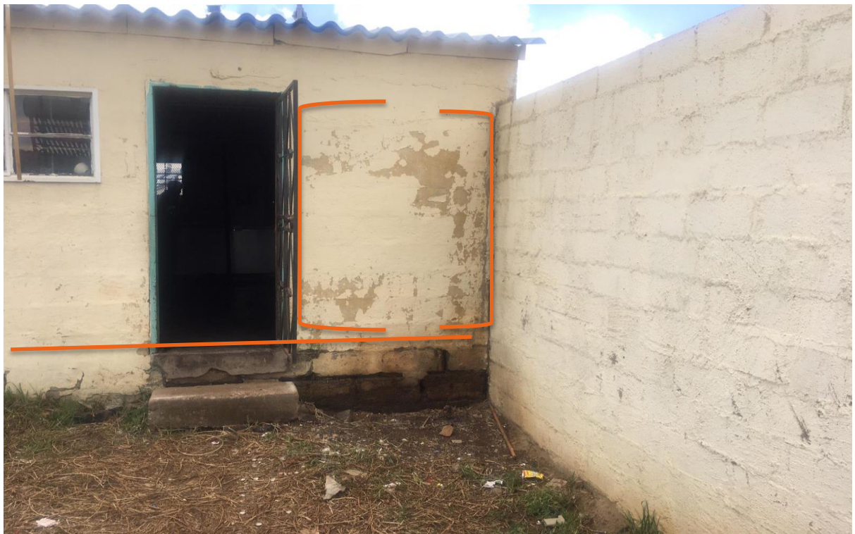
Figure 8 : View of the dilapidated foundations peeling off paint showing lack of maintenance
