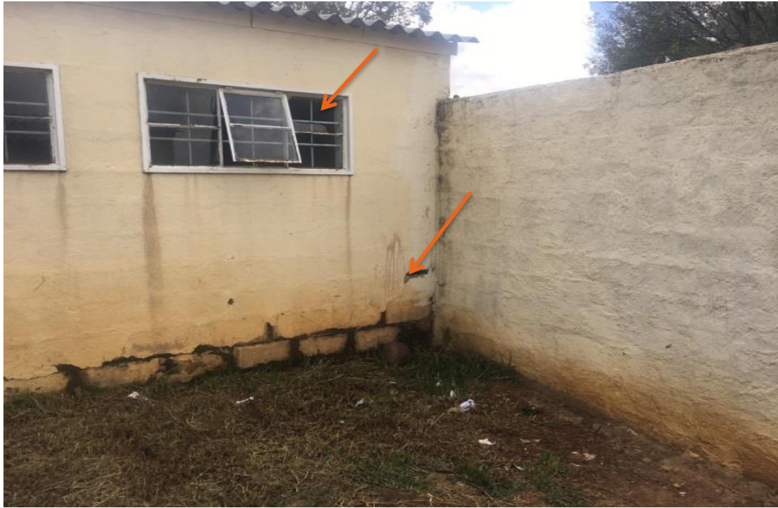
Figure 9: View of the disturbing cracks and broken windows on some of the buildings on site
