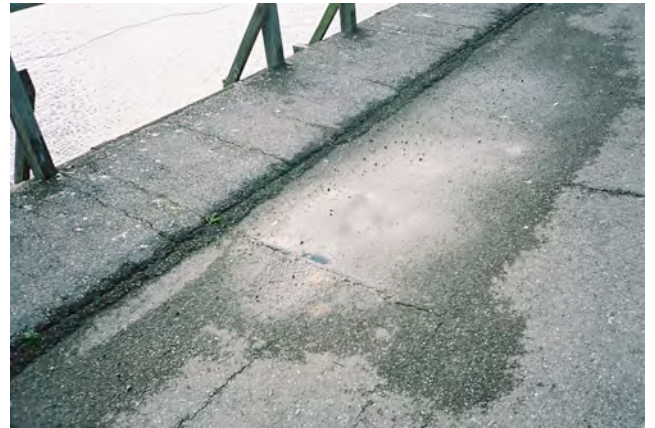
Ponding to surface
