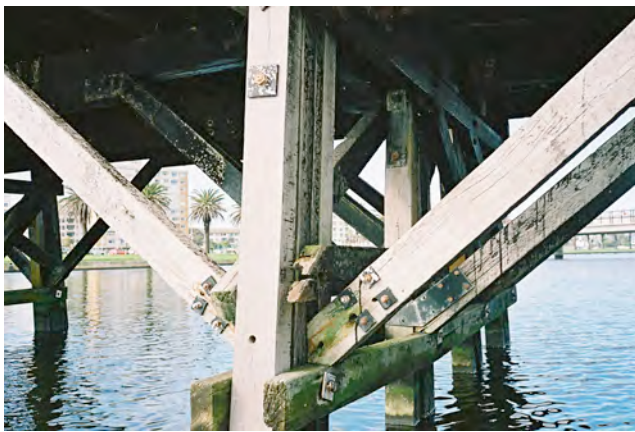
Deteriorating ends to structural member
