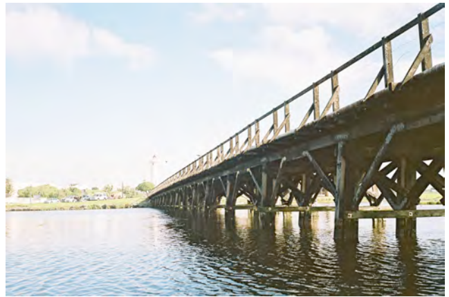
General view looking north west Note slight visible deflection
