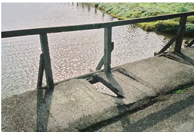
Holes to decking at east end
