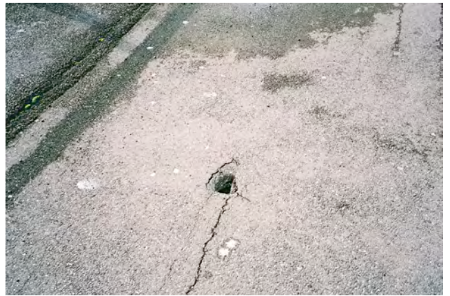
Hole in decking
