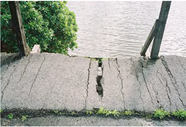
Sagging and collapsed decking to west end
