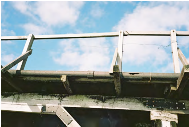
Defunct service pipe along bridge
