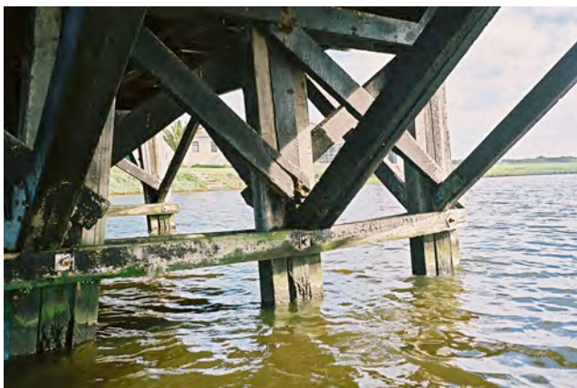
Split and sagging members
