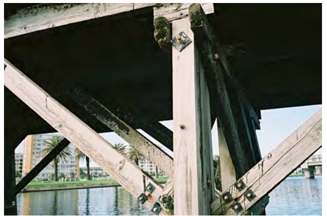
Note missing nut and washer to bolt
