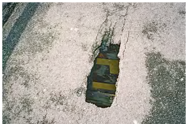
Hole to decking
