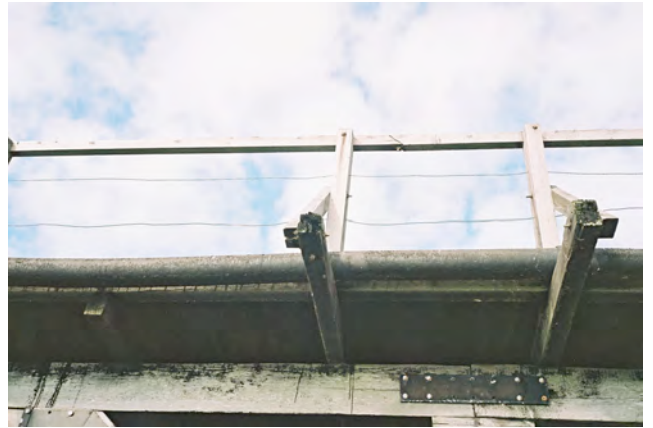
Deteriorating horizontal supports to handrail
