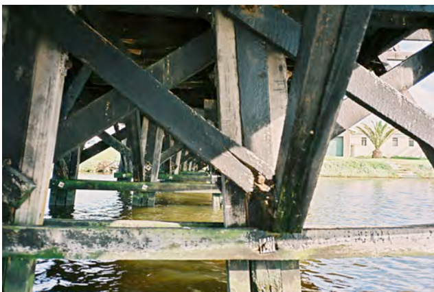
Split end to cross-bracing
