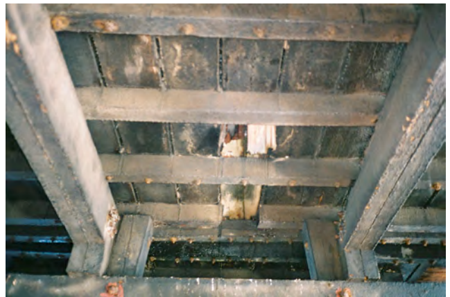
View to undercarriage. Note mould growth, collapsing decking
