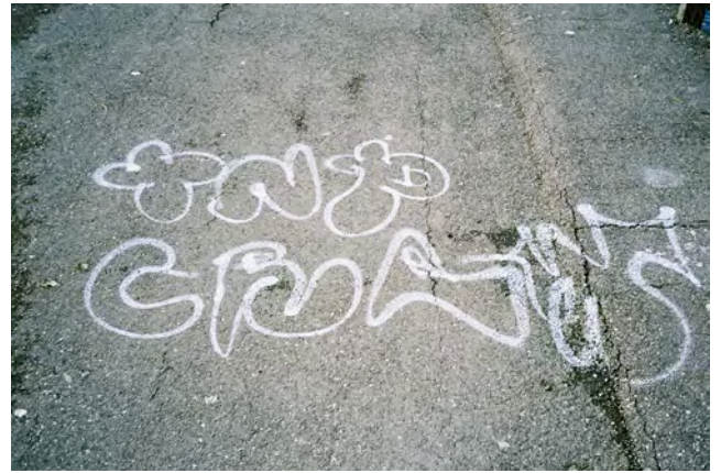
Graffiti to bridge deck
