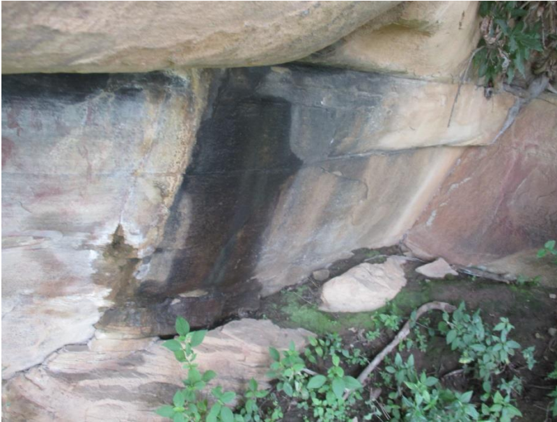
Figure 16: Seepage is present causing accretion over the parent rock and paintings (Mbatha, S. 18 January 2021, storage: The Institute).
