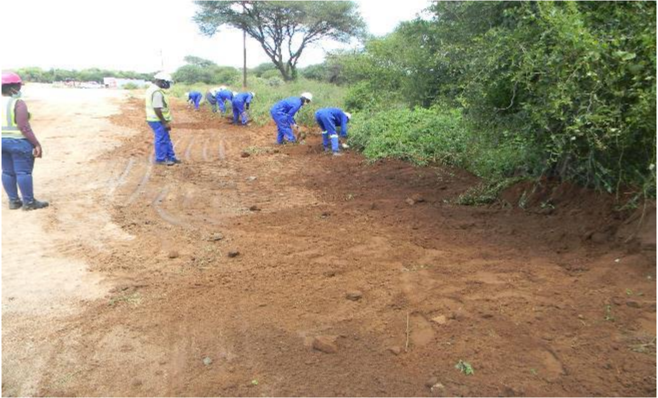
Plates 6: View of construction workers working along the access road reserve (Author 2021)
